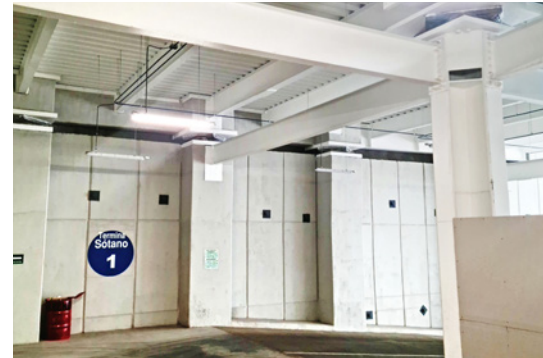
Four of the total 34 installed SIP®-A bearings on top of the support columns. Visible at the bottom is the descent to the underground car park.
