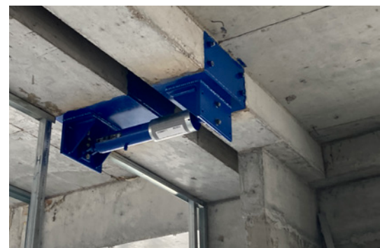
One of the four hydraulic dampers to protect the narrow building core against tilting.
